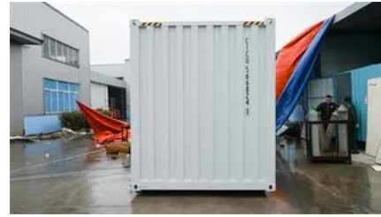
The working principle of the power storage cabinet
