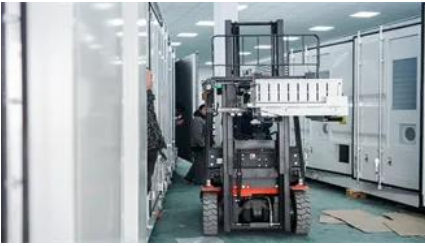
Battery Cabinet, Battery Storage Cabinet, Battery Bank
