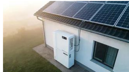
600kW Photovoltaic Battery Cabinet vs. Photovoltaics
