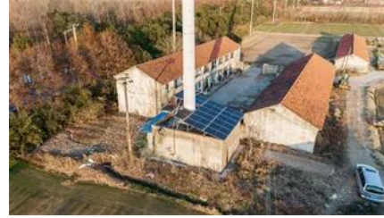
Photovoltaic Micro-station Energy Cabinet
