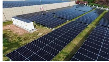
Communication site energy cabinet management system
