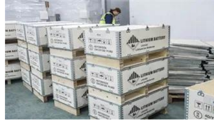
CATL EnerC+ 306 4MWH Battery Energy Storage
