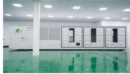
Bhutan Energy Storage Power Station Battery
