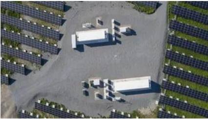
Outdoor Energy Storage Cabinet - solaryyy
