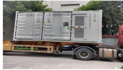
Mega power storage utility operational in northeast China
