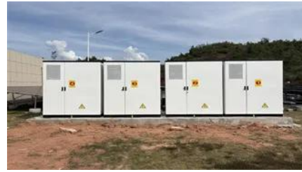
Outdoor Communication Energy Cabinet With Wind Turbine
