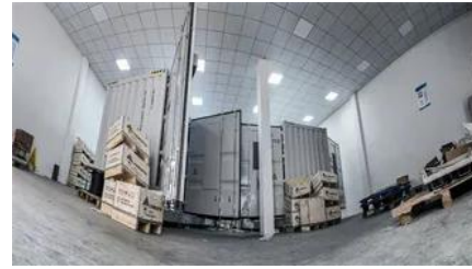
No.1 Capacity Solar Container , Solarabox
