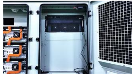
Solar Company in Phoenix AZ , Capital Energy Solar Experts
