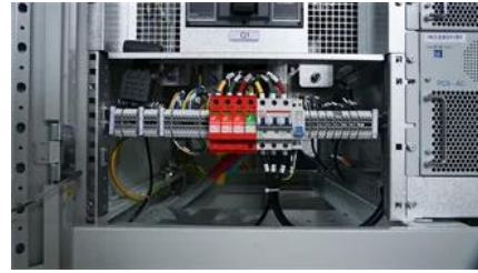
Solar container lithium battery power station in Cape-Town
