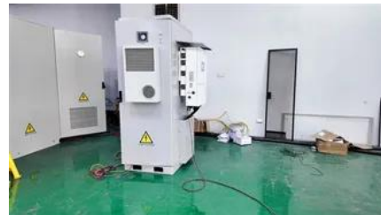
Li-Ion Battery Storage solar power system.
