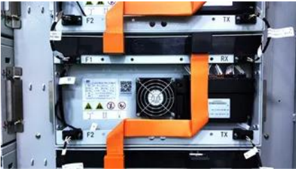
Containerized energy storage , Microgreen.ca
