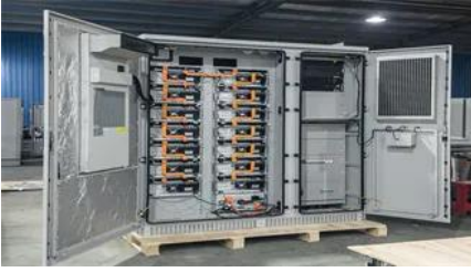
Utility-scale battery energy storage system (BESS)
