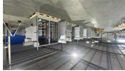
Port Moresby Wind and Solar Storage: Powering a Sustainable Future
