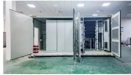
5MWh Battery Storage Container (eTRON BESS)
