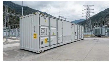
2MWH Container Solar Battery Storage System -
