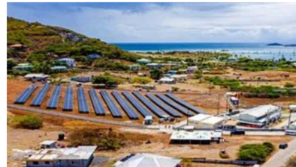
Oceania Photovoltaic Energy Storage Container Wind-Resistant Type
