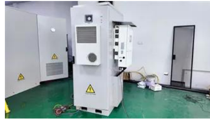
Outdoor Telecom Enclosures & NEMA Cabinets , AmProd
