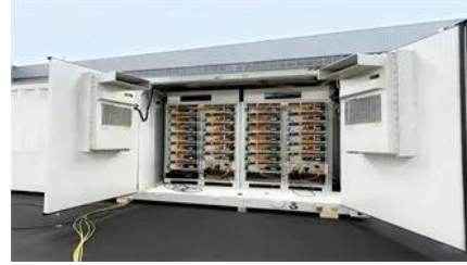
Huawei Northern Cyprus Distributed Energy Storage Project
