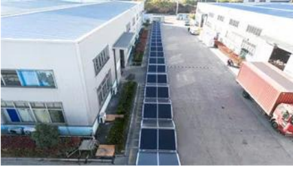
Niue 5G solar container communication station hybrid energy
