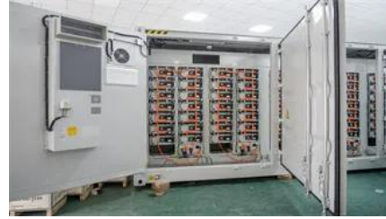
Niger Demonstration solar container communication station
