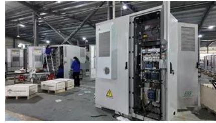
BESS Battery Energy Storage Cabinet 200kWh Barbados
