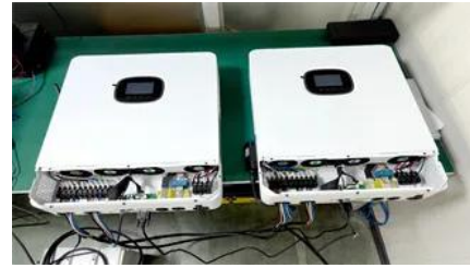
Latvia energy storage: Impressive 2024 battery projects
