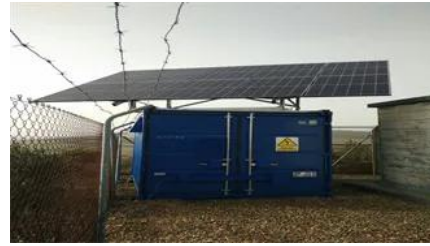
15mwh solar energy storage cabinet cabinet used on baghdad island
