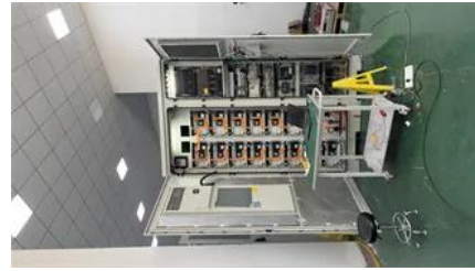
Outdoor Battery Cabinet - Premtel Systems Sdn Bhd
