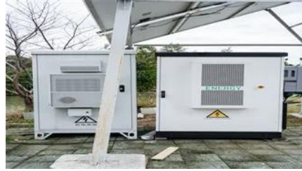
Battery Energy Storage System in India , Powering RE future
