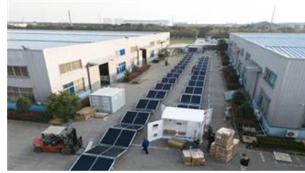
5g solar container communication station wind and solar
