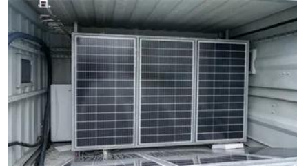
Honiara 2mw Energy Storage Smart Microgrid
