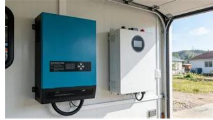
UAE grid-connected wind power generation system
