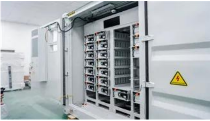
Energy storage container, BESS container
