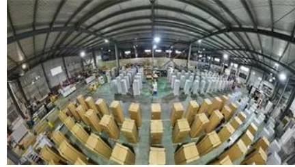
Finland's largest Battery Energy Storage System
