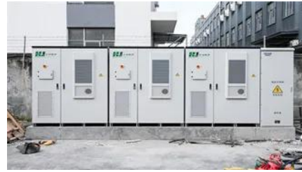
2025 Single-Family Battery Energy Storage System
