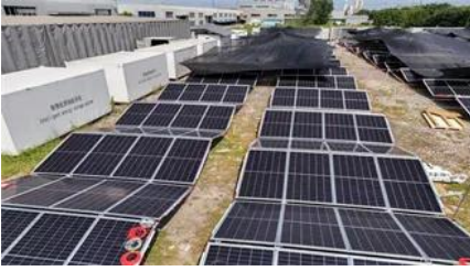
OUTDOOR MODULAR CABINET , Solar Power Solutions
