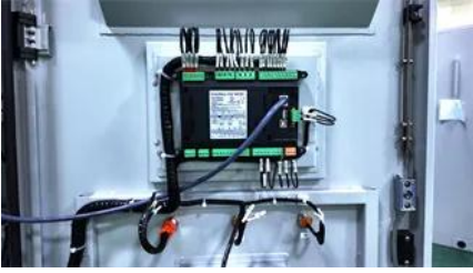
EK flywheel energy storage production site
