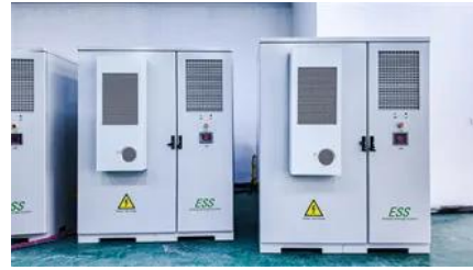
Outdoor Cabinet Bess Lithium Battery 100kwh Dominican
