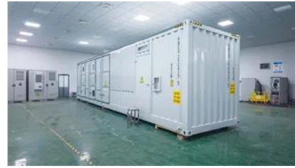
200 kWh Battery Energy Storage System , BESS Cabinets
