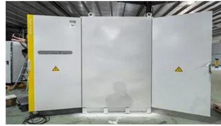
Circuit Breaker & Automatic Transfer Switch , Relay & Contactor
