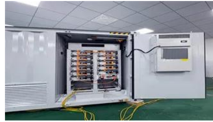
Koten Safety Breaker In China , HALKIDIKI BESS
