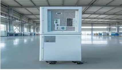
Benin Energy Storage Cabinet Battery Production
