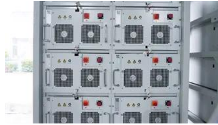
Battery Cabinet, Battery Storage Cabinet, Battery Bank Rack
