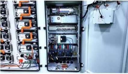
Telecom Battery Backup System , Sunwoda Energy
