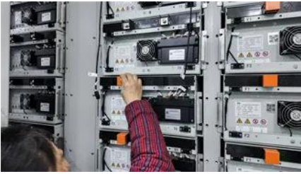
Site Power Solutions & Facility . Huawei Digital Power
