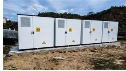
Solar container communication station inverter grid-connected
