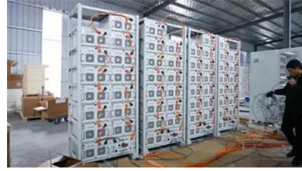
Customized energy storage container power station in Angola
