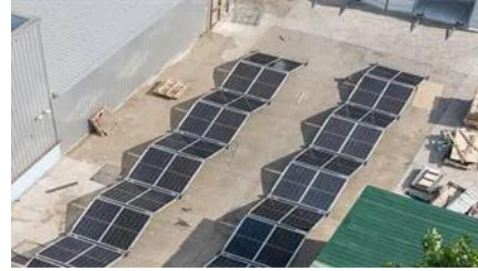
Mobile Solar PV Container , Portable Photovoltaic
