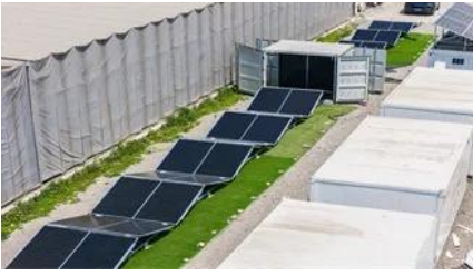
Bess Solar Battery Energy Storage System 5mwh
