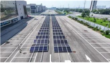
PORT OF SAN SALVADOR ENERGY STORAGE , WALMER ENERGY
