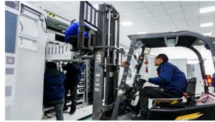
Kyrgyzstan Osh Energy Storage System: Powering Central Asia with
